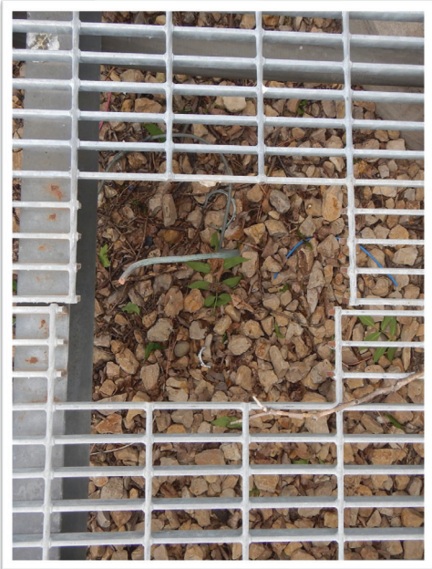
Hole in Platform
